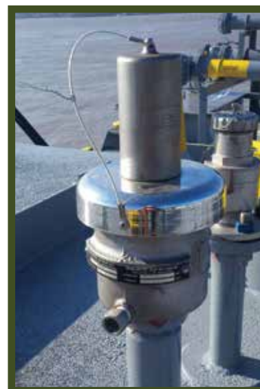
2.5" Equate PV Valve mounted on stand pipe next to 2" Sampling Ball Valve.
