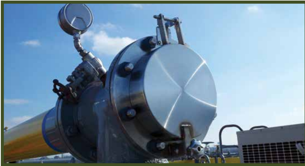
Typical Vapor Headers with ERL Vent Header Sight Glass and ERL Model 505 Pressure/Vacuum Gauge.
