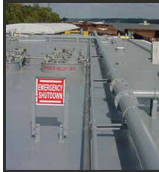
Emergency Shutdown Sign and Frame mounted next to main vapor line.
