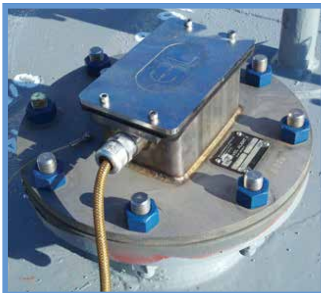
LEVEL ALERT II High Level/Overfill Liquid Level Alarm Sensor Installed.
